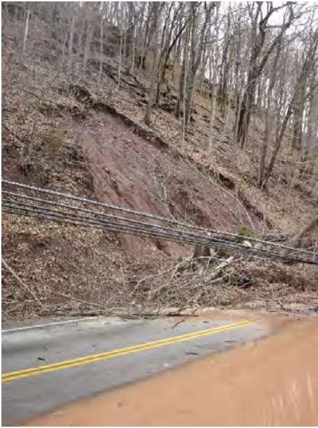
Figure 13. April 2005 landslide one mile south of Milford in Holland Township, Hunterdon County. Photograph courtesy of Hunterdon County Road Dept.
