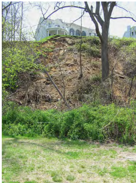
Figure 4. Landslide in Highlands Borough, Monmouth County, triggered by heavy rains from the April 15-16, 2007, northeaster. Photograph by S. Stanford, N.J. Geological Survey.
