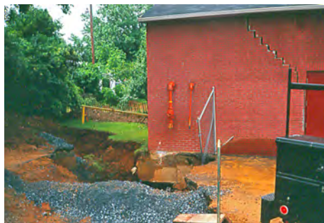
Figure 13. Water-treatment plant building in Warren County damaged by a soil collapse sinkhole (Greg Herman).
