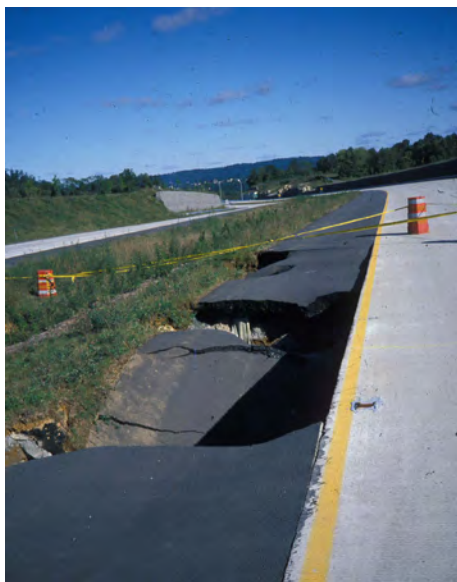
Figure 14. Soil collapse sinkhole on Interstate Route 78 prior to the opening of the Phillipsburg bypass section, Warren County (NJDOT).
