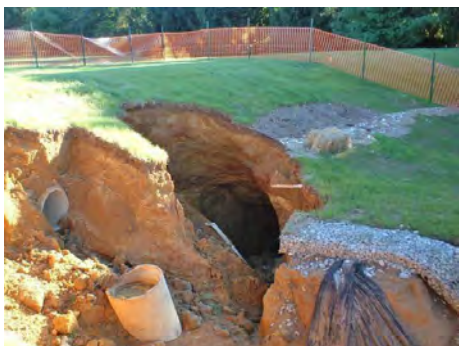
Figure 12. Excavation showing a large soil void sinkhole, Greenwich, Warren County. The broken storm sewer pipe is three feet in diameter (Joe Fischer).
